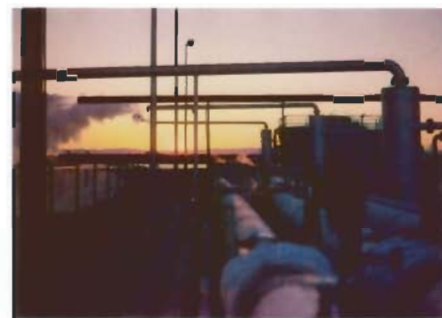
Barber-Nichols 500-kW geothermal power plant.
